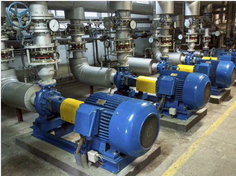
(a) Electrical motors in an industrial environment
