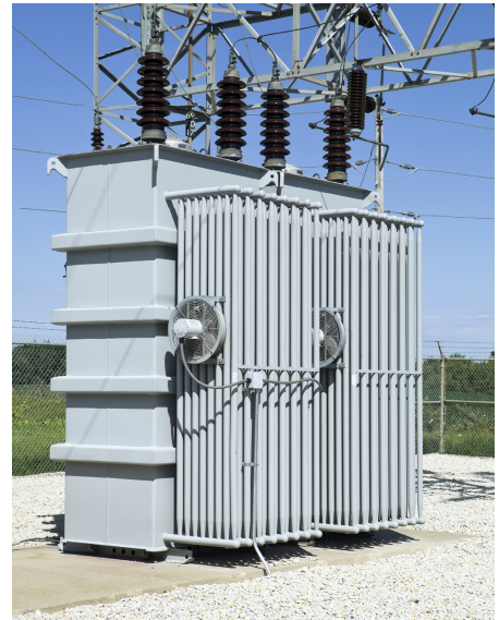
(b) Power transformer in an electric substation
